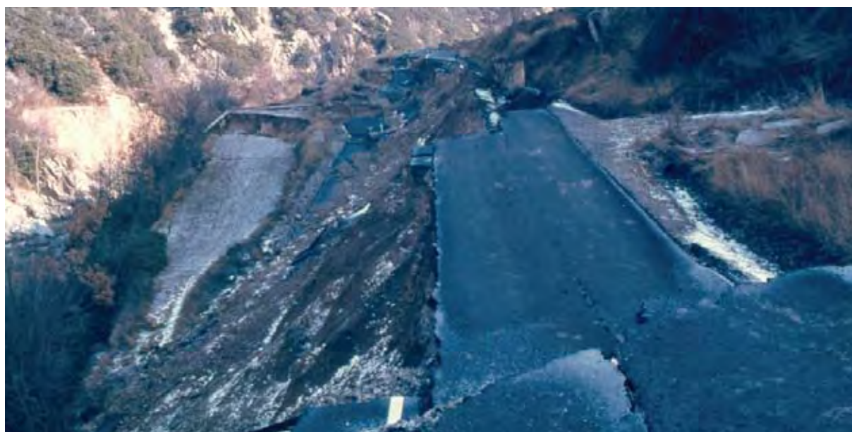
Destruction of the road N-260 by a landslide. El Pont de Bar during the heavy rains in November 1982 (Photo J.M. Vilaplana).
