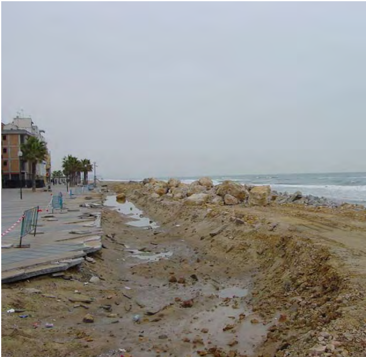
Effects of the easterly sea storm in 2003 on the seafront avenue of Torredembarra. (Photo J. Guillén).
