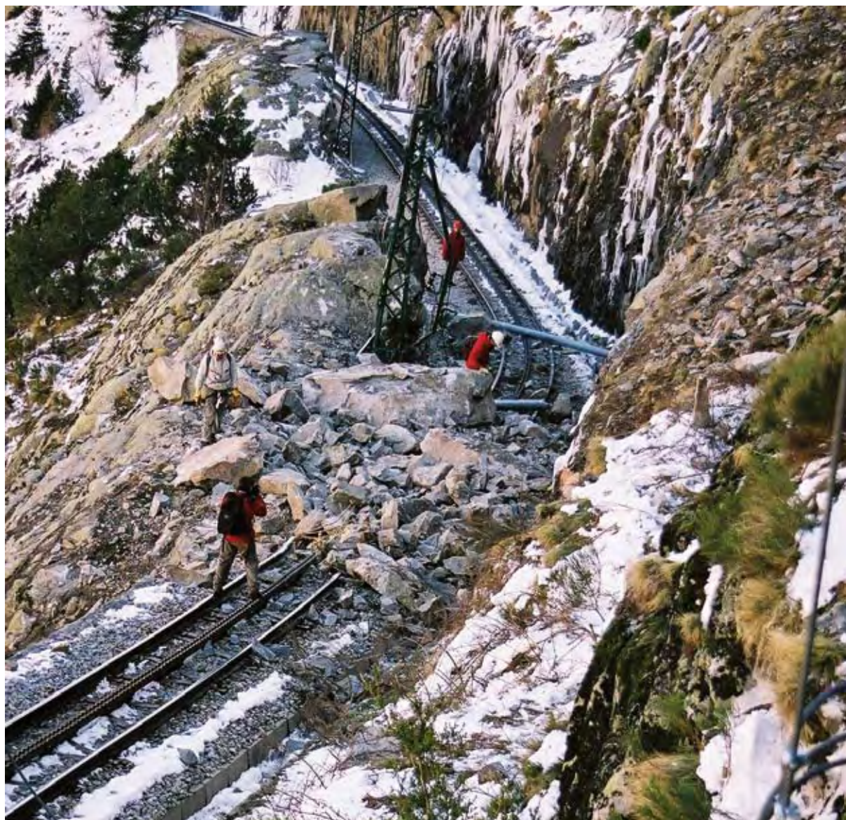
Damages to the rack railway in Vall de Núria caused by a rock landslide in 2003. (Photo J.M. Vilaplana)
