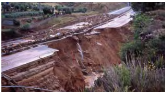
Damages to the road N-II in Esparreguera during the rain of June 2000. (Photo M.A. Marquès)
